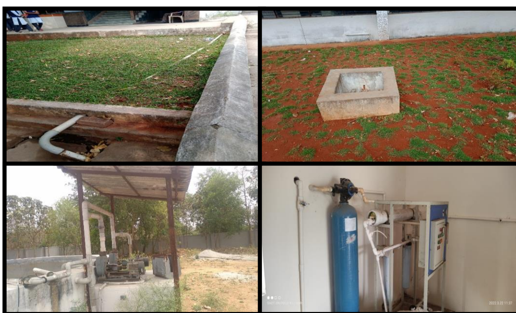
Water supply units and treatment facilities at ACE, Hosur, Tamilnadu.
