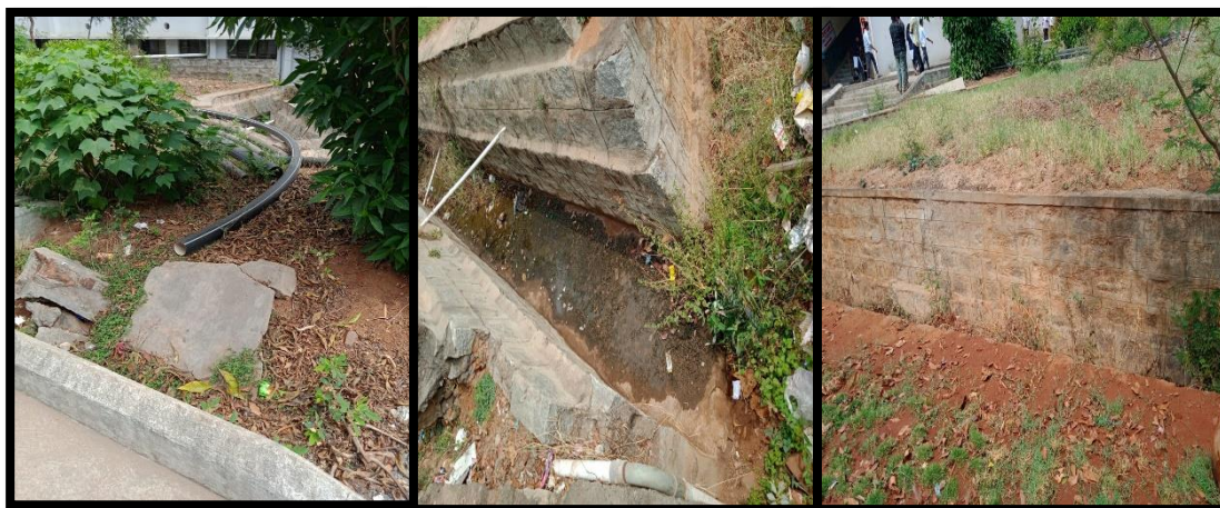
Water management facilities in ACE, Hosur, Tamilnadu.
