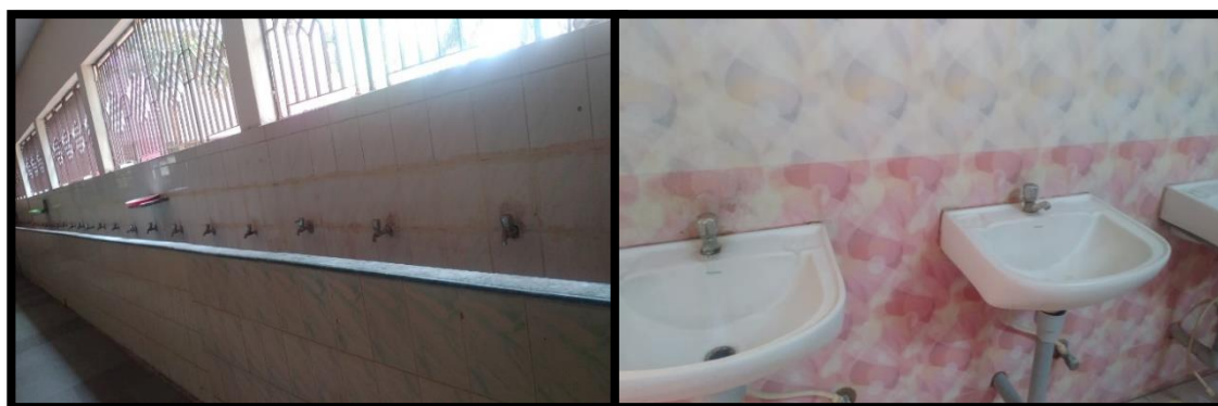
Proper maintenance of taps in each floor in ACE, Hosur, Tamilnadu.
