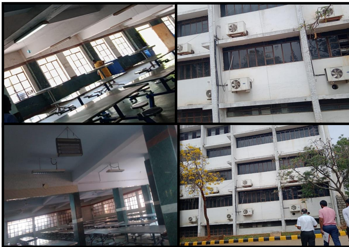
Ventilation and Exhaust system Facilities in ACE Buildings
